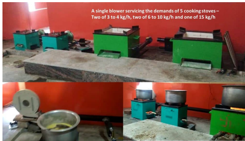
Figure 33: Two of 3 to 6 kg/h, two of 6 to 10 kg/h VEBCOD systems operating with a single blower for community cooking
