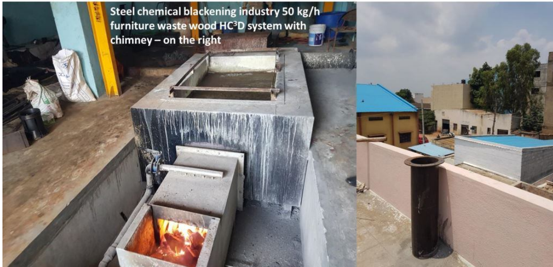
Figure 28: The HC 3 D system with chimney operating at about 50 kg/h with wood cuts from a furniture industry in a blackening unit for metal parts
